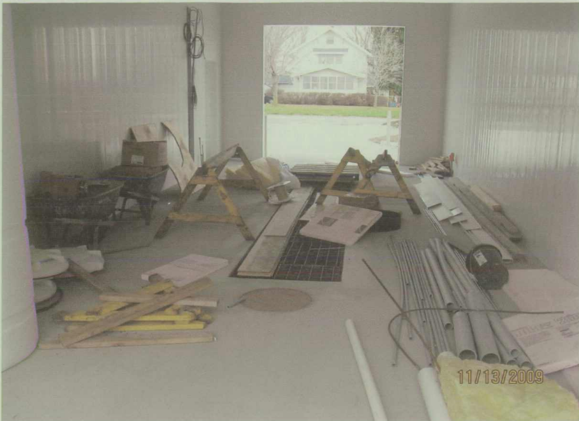
Photo 7. Interior view of one of the unfinished wash bays in the new car wash, showing construction materials.
