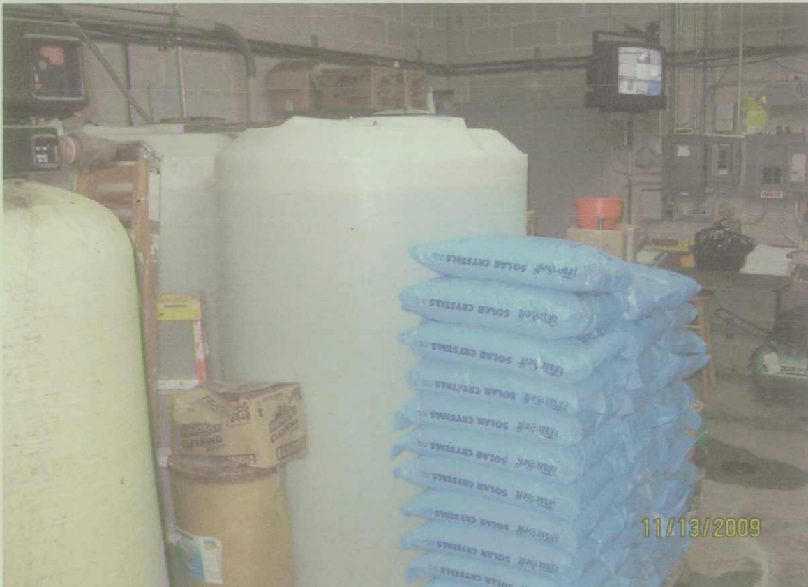
Photo 10. An equipment room located near the south end of the original car wash, showing bags of water treatment chemicals and water storage tanks.
