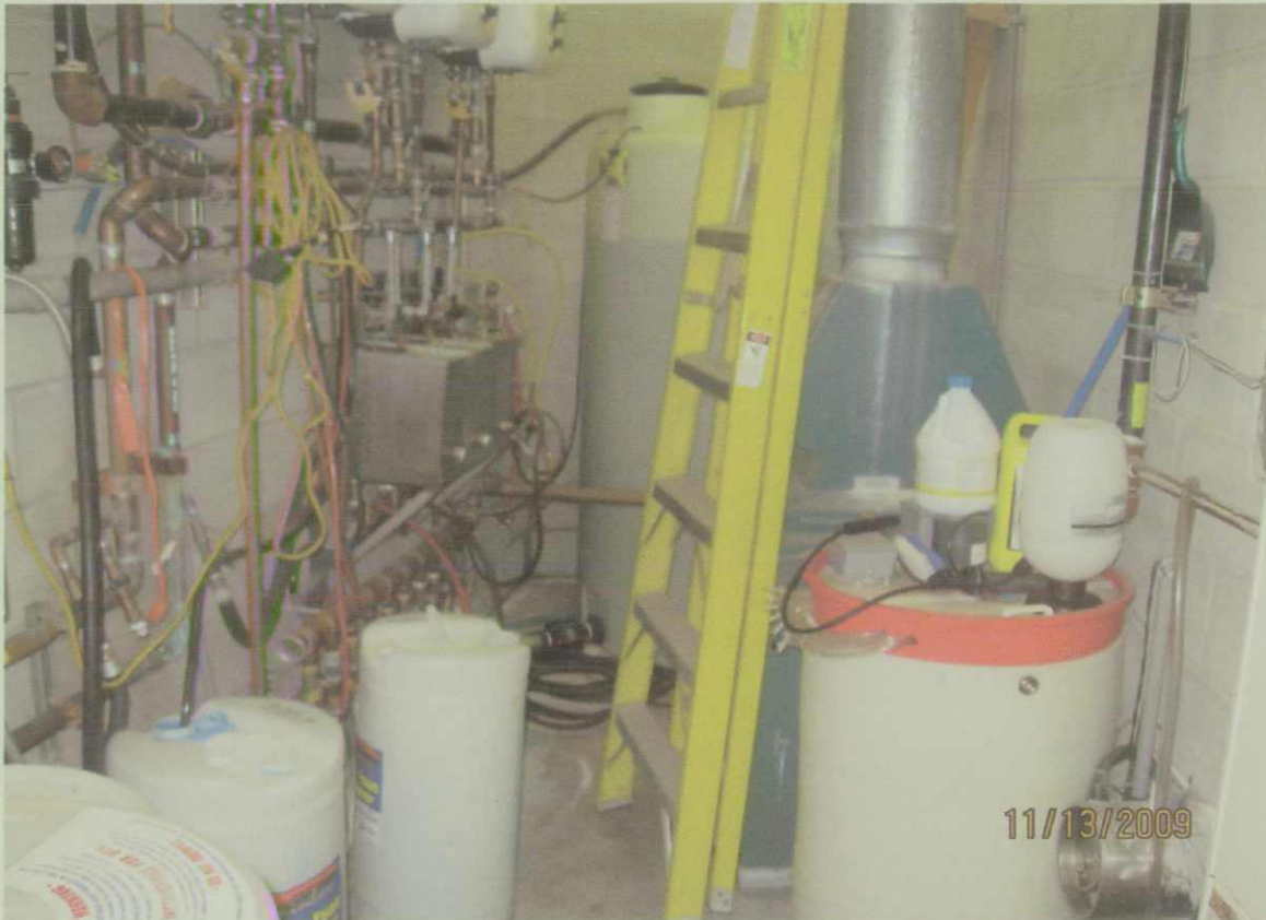
Photo 9. An equipment room located near the north end of the original car wash, showing car wash soaps and water treatment storage tanks.
