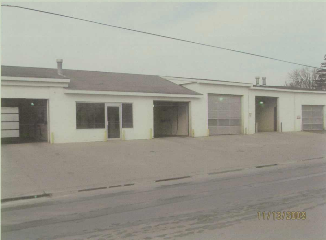
Photo 6. West-northwest view of the original car wash located on the east side of the property. Fifteenth Street appears in the foreground.
