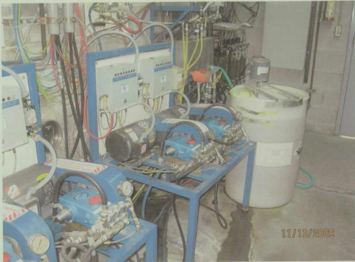
Photo 11. View inside the south equipment room of the original car wash showing pumps and a drum of car wash soap.
