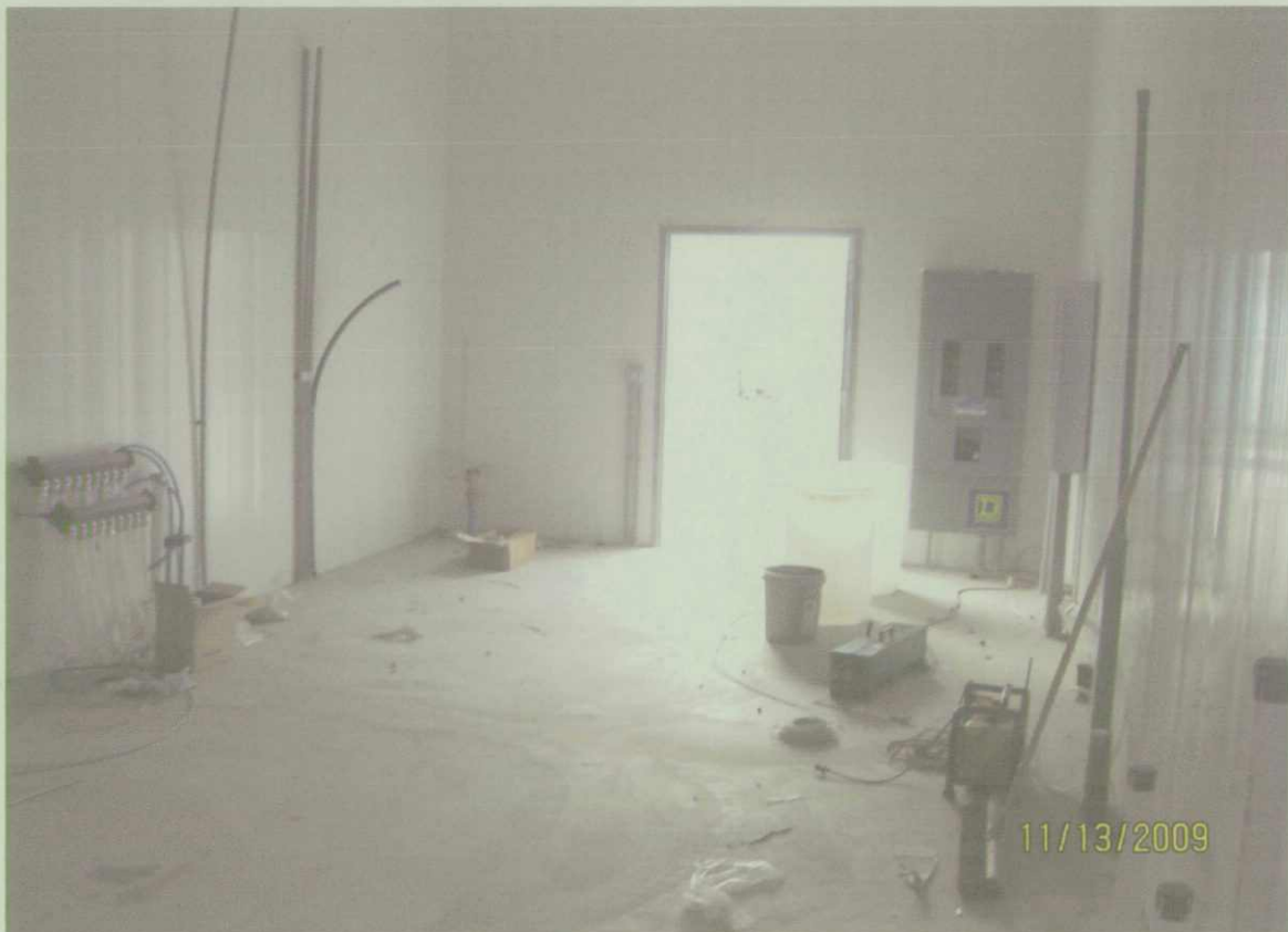
Photo 8. An unfinished equipment room located in the middle of the new car wash.
