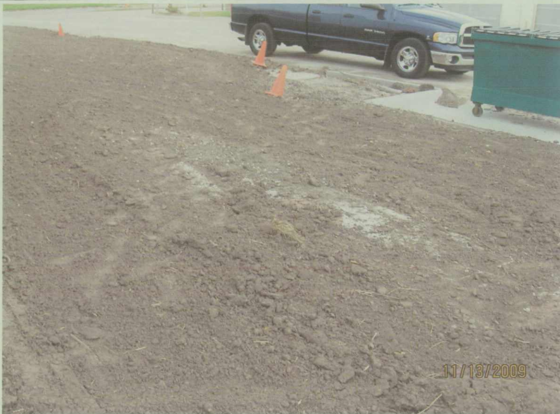
Photo 5. Northeast view of the ground located southeast of the new car wash where three underground water treatment storage tanks are buried.
