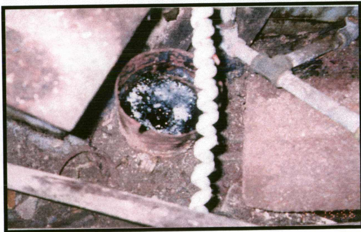
Oil "sludge" next to barrel of unknown content in boiler room.
