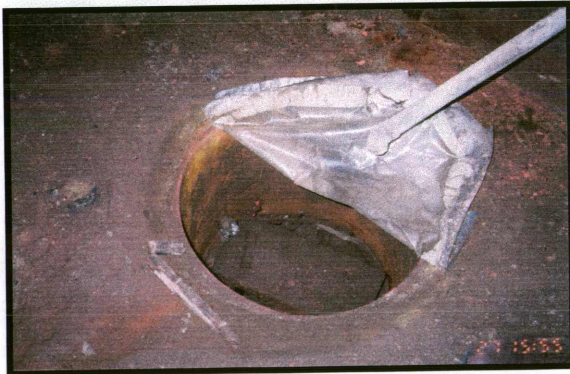
Sump pump in boiler room.
