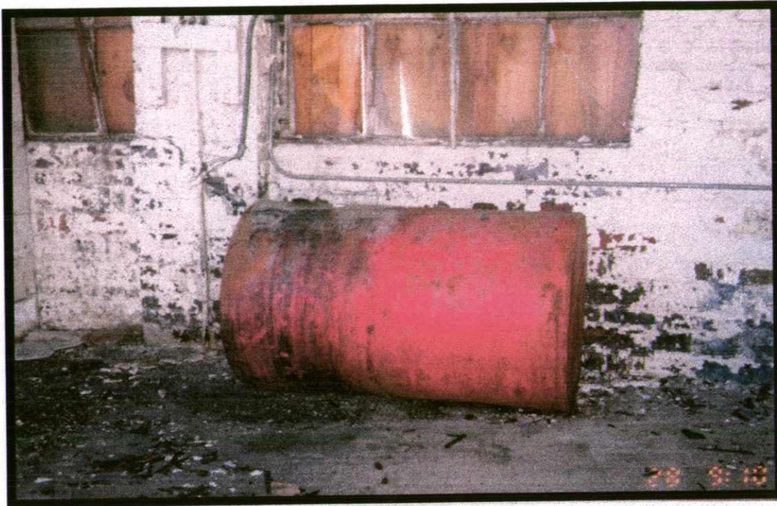
Above ground storage tank with noticeable staining along south wall of the south-west portion of the site. Contains approximately 4 inches of petroleum product.
