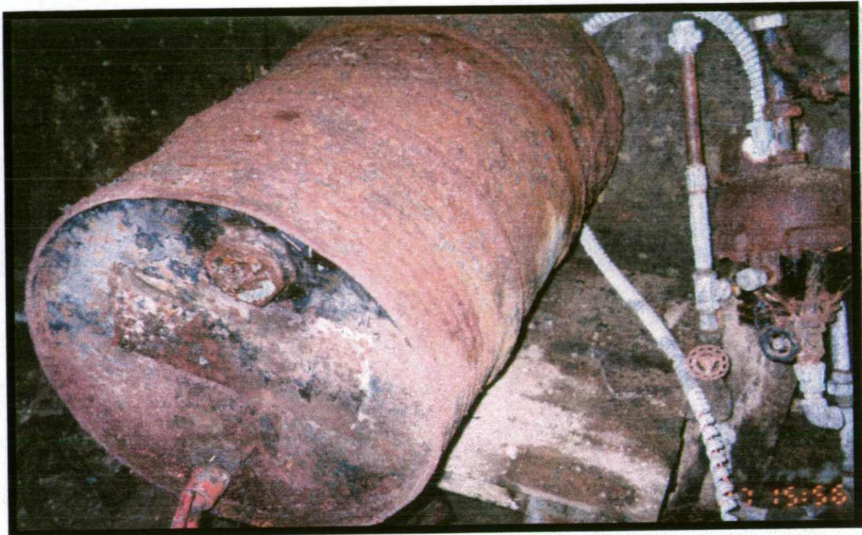
Heavily corroded 55 gallon barrel of unknown content (some kind of fuel as noted on barrel) with spigot - located in boiler room.
